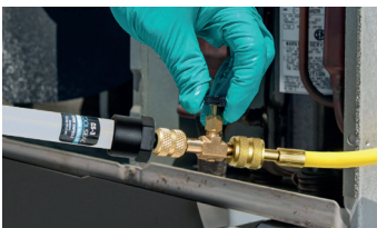
Charge inline with refrigerant
